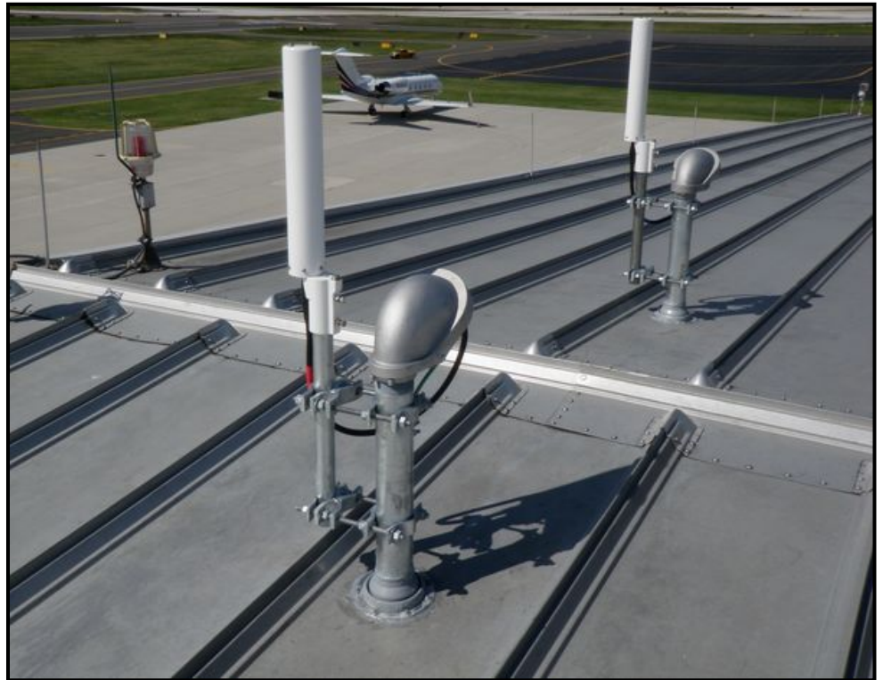
1090 and UAT Antennas
